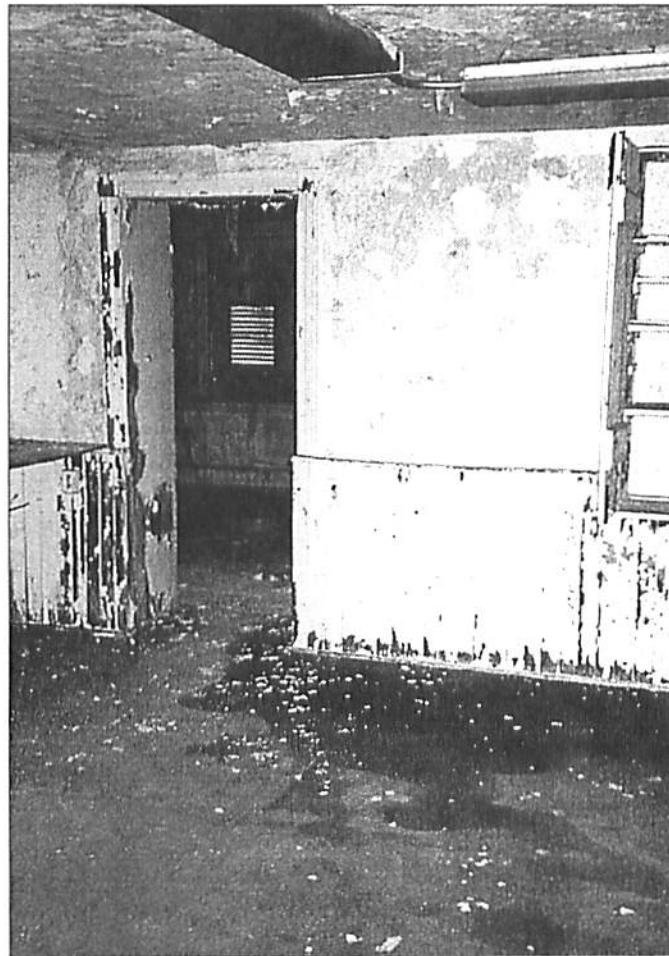
Figure 17. Water has infiltrated the interior of the building through the window louvers and wet the existing carpeting and flooring. Damp wood is appealing to insects and should be avoided.
