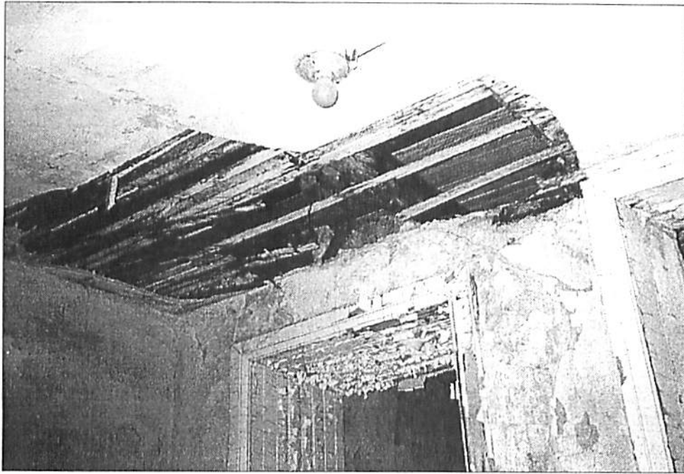
Figure 19: Water damage has caused sections of ceiling plaster and lath to collapse.
