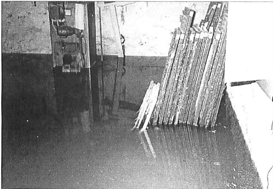
Figure 20. At the time of the survey, there was eleven inches of standing water in the basement. A sump pump and alarm system should be installed in the basement to prevent further water damage to the structure.
