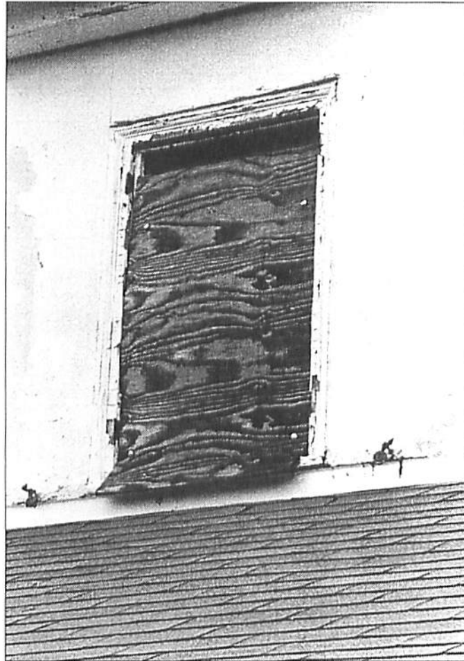
Figure 15. View of a plywood window panel that has warped and slipped. The existing panels should be replaced with painted, marine-grade plywood panels if the building is to remain vacant for an extended period of time.
