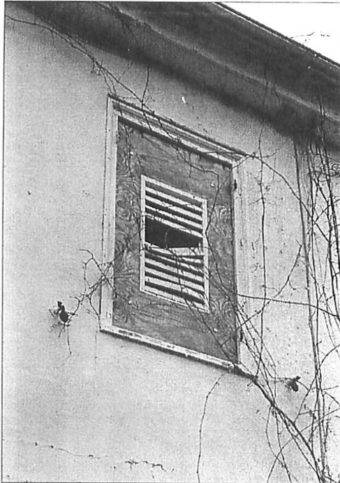
Figure 16. View of a broken louver on one of the plywood window panels. Replace plywood panels.
