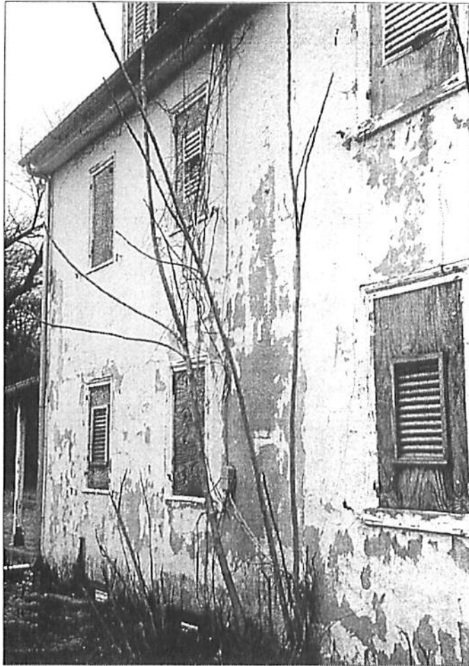
Figure 13. The window and door openings on the Murphy House were sheathed with vented plywood panels. This was an appropriate stabilization procedure.
