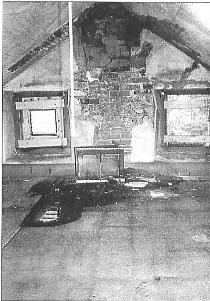
Figure 18. View of a chimney base at the attic level. The chimneys on the house should be capped and repointed and their flashing checked to prevent further water from entering the building through them.
