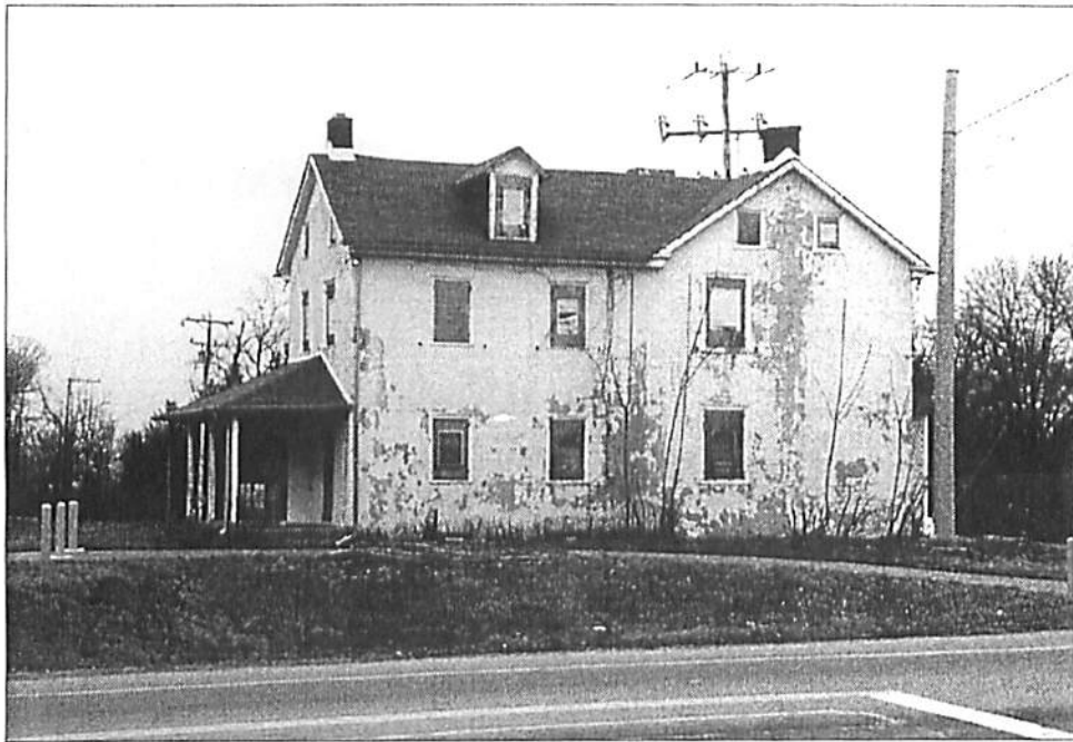
Figure 5 West elevation, the George Murphy House. The stone portion of the structure is to the right of the photograph, the frame ell is to the left.
